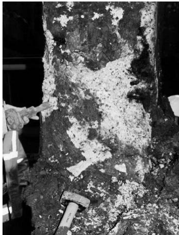
Figure 2.12. Severe sulphate attack in a bridge structure exposed to wet, pyritic clay fill
